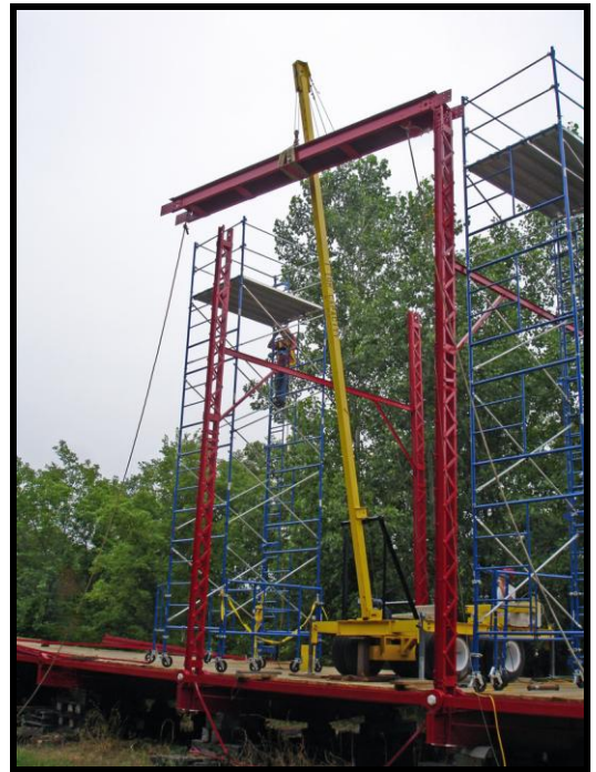
Gin Pole lifting a top chord section on the Charlotte Highway Bridge.
